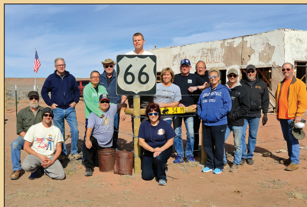
Volunteers came from all parts of the U. S. to help with the roof replacement during the second phase.
